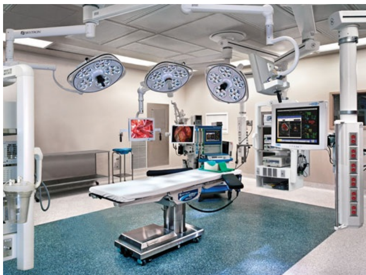
Integrated operating room, Skytron
